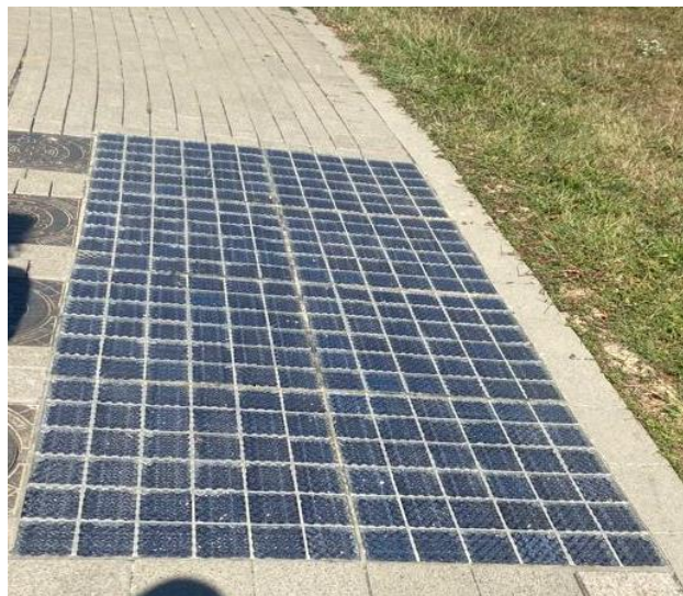
Figure 3.3 Silicon Wafer RIPV with capacity (0.304 kWp) ,Solmove (38 wp),8 modules installed
